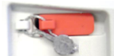
Locked with Wire Seal
